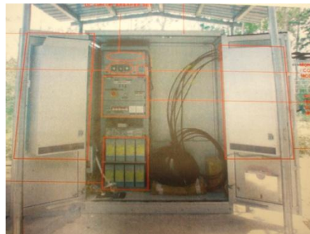
DC SWITCHMODE RECTIFIER (SMR) COMPLETE WITH BATTERIES
